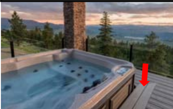
Removable patio boards for access to equipment
