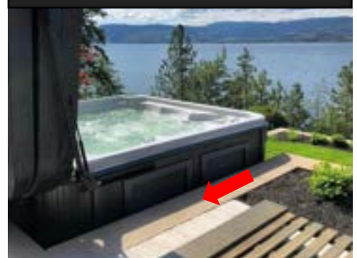
Low wall under the door screws – low wall located 4 inches from the spa
